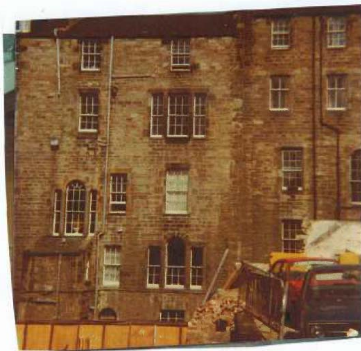
This 1981 photograph shows the demolition of an old building to the rear of No. 56 Frederick Street, which Balfour & Manson had purchased; once the site had been cleared, the present Cashroom was built on it.
